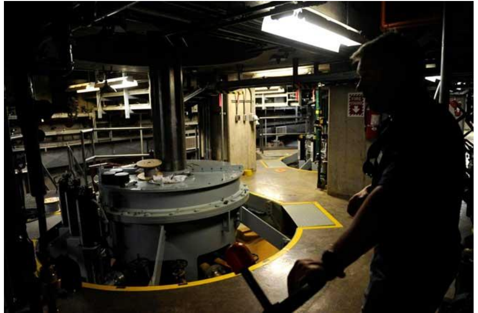
Windy Gap pumps on Colorado River
